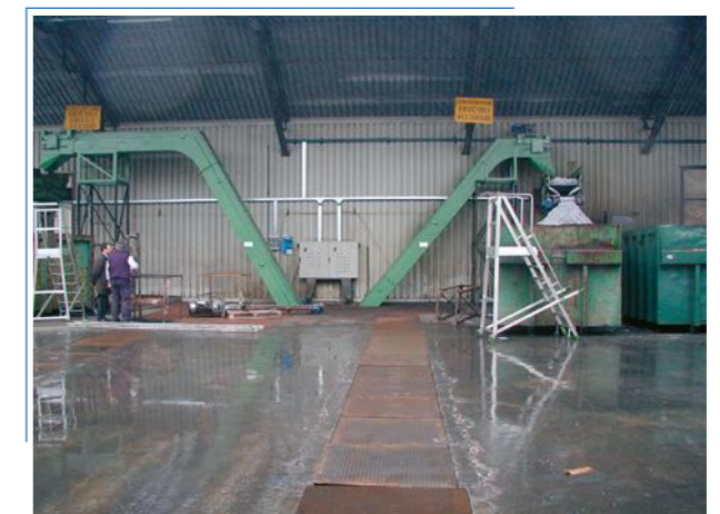
Aluminium conveying line
