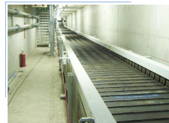
In-ground line for offcuts
