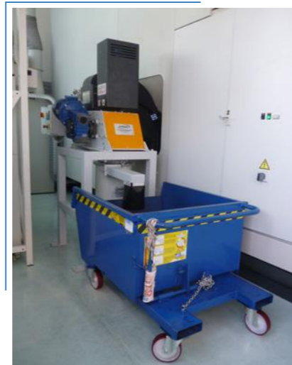
Shredding and spinning unit under the machine tool conveyor
