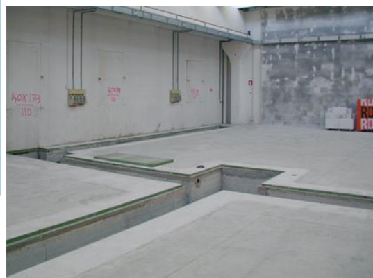
Detail of in-ground lines
