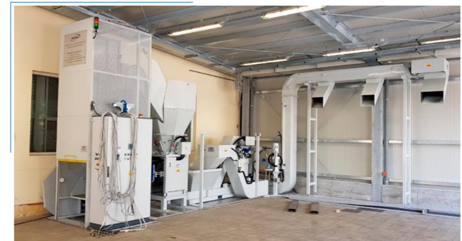
Minisystem with skipoist, crusher and discharge into container
