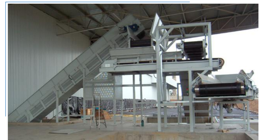
Aluminium and steel offcuts conveying line
