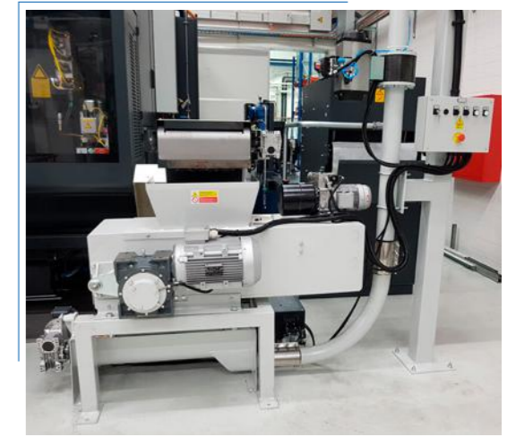
Vacuum station equipped with grinder
