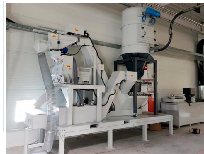
Vacuum plant discharging into a spinning system
